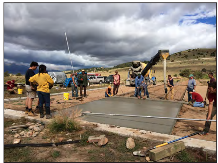
Staff and volunteers help pour and level concrete for the fire barn floor. (Photo by Gayle Nosal)
