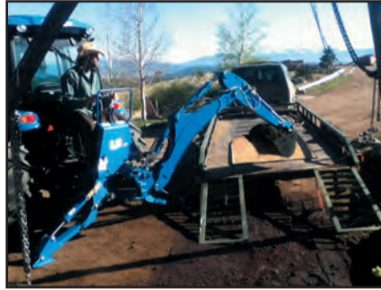
Right: Kent excavates a drainage system with the new tractor. (Photo by Hoyt)
