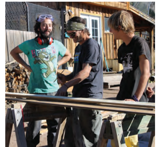
Marco Valera, Christian Hatt, and River Dougherty work on insulating an office cabin roof. (Photo by Hoyt)
