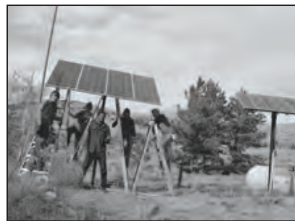
A group of volunteers install a new solar panel under the windmill at the farm
