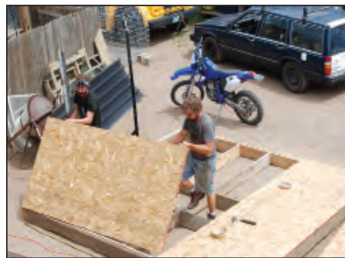
Volunteers Travis and Andrew constructing a new shed made out of recycled materials
